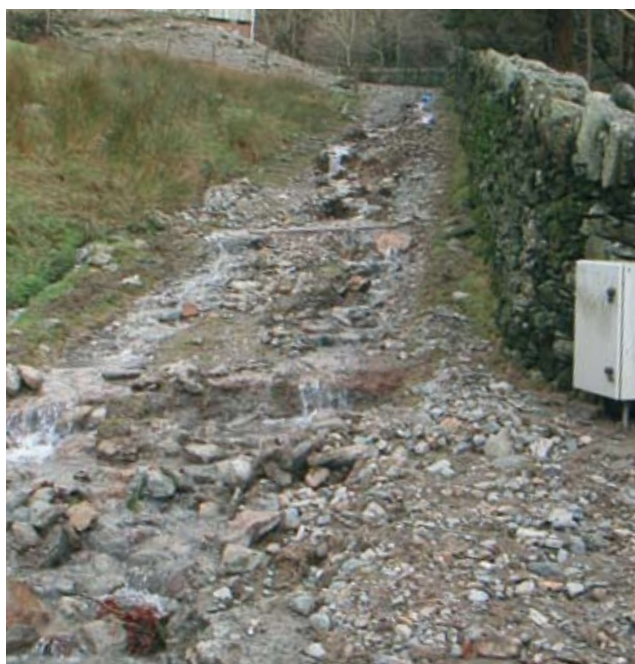
Road damage at the top of Rydal Hill, January 2005
