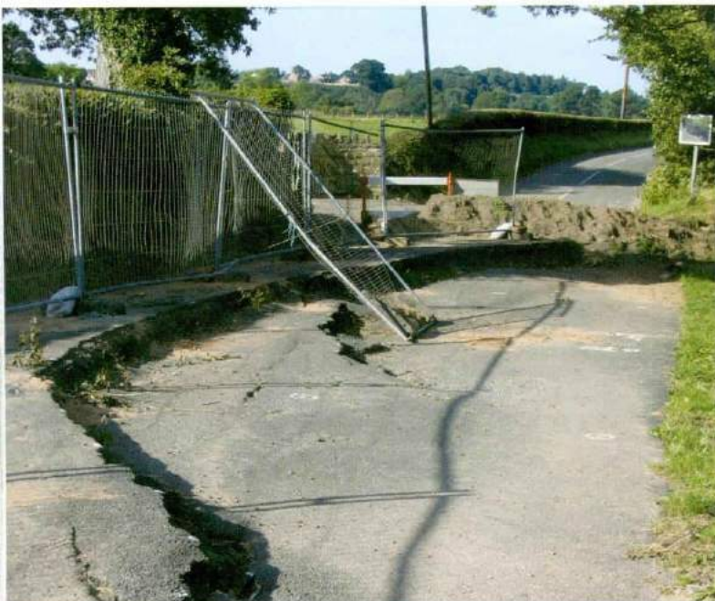
Subsidence on B6263, Wetheral
